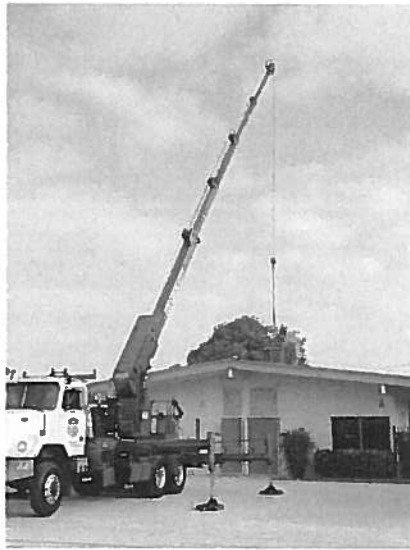
Pictured here: Air-conditioning is being installed at Barker Elementary School, just in time for the start of the school year!
