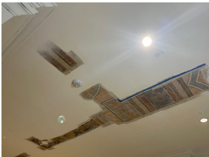
Frescoes in the lobby were also plastered over; here's a view of what can still be seen. Not all the ceiling can be recovered
